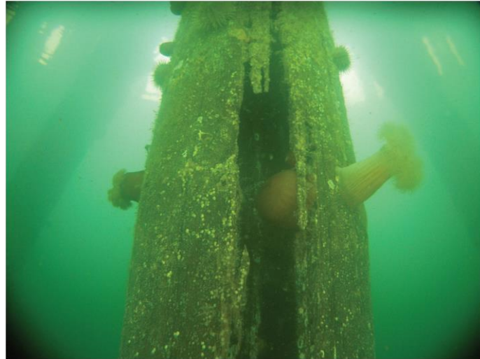
Fig. B-20. Underwater photograph showing hollowing of the interior of a timber pile from Teredo Source: Courtesy of Marine Solutions, Inc., reproduced with permission.
