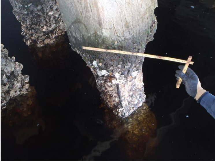
Fig. B-9. Reinforced concrete pile with loss of section below the high tide level Source: Courtesy of Marine Solutions, Inc., reproduced with permission.
