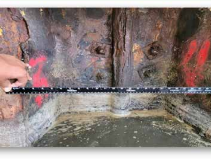
Corroding Sheet Pile Wall
