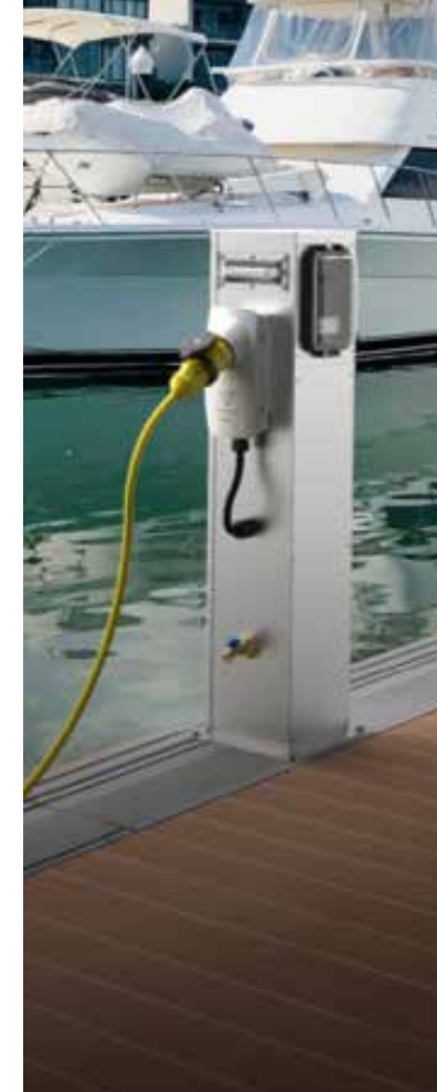
VoltSafe Smart Marina Shore Power Solution
