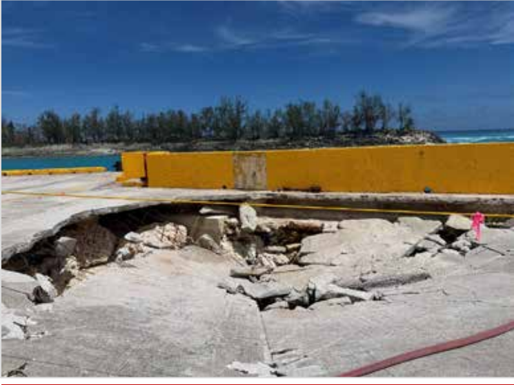
Large Cavity at Berth 2
