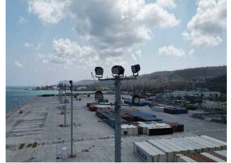
Damaged Dock Lights
