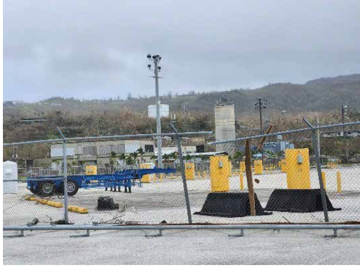
Compromised Chain Link Fence
